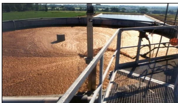
Figure 10. Biological nitrification/denitrification tank (VCM, n.d.)
